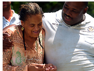
SARAH GRILE Indian River sheriff's deputy Teddy Floyd gives Martha Rainey a hug before her house in Fellsmere is demolished on Saturday. A new house will be built for Rainey in October through the Indian River County Health Department's Protocol for Assessing Community Excellence program, which identifies blighted areas in the county and meets with residents to find solutions to the problems.
